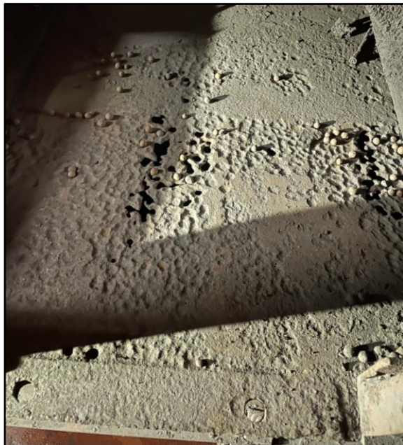
Example steel in poor condition
