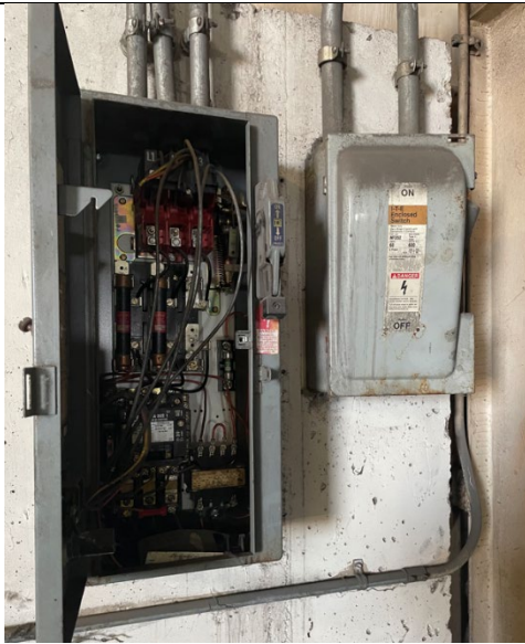
Photo 2.4.2.9 Close-up of starter/disconnect for furnace of south end of Warehouse A
