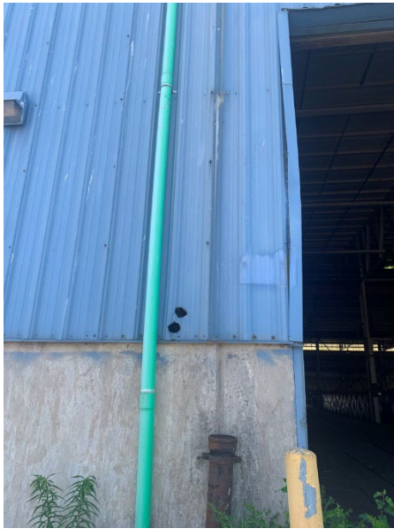
Photo 2.1.1.1.9 Damaged trim at jamb of overhead door.
