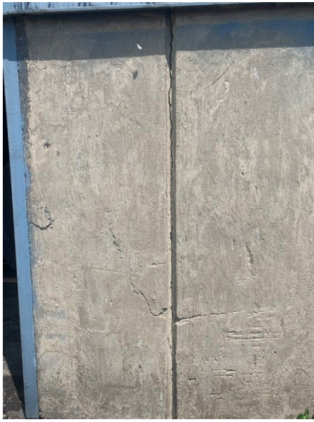
Photo 2.1.1.1.1 Vertical crack located at the control joint. Other minor cracking each side of the joint. Cracks should be routed out and repaired.
