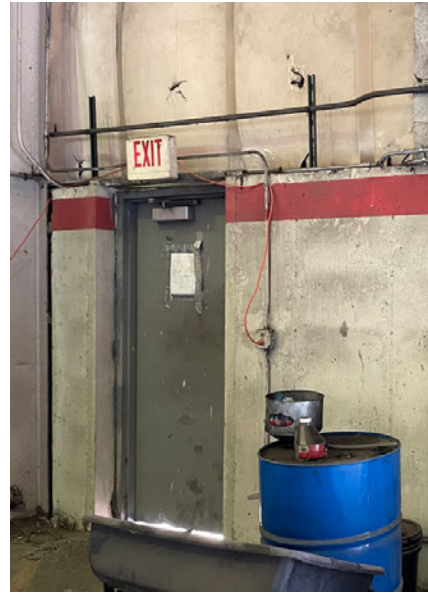
Photo 2.4.4.2 Absence of fire alarm horn/strobe and manual pull stations noted at exits at Warehouse A
