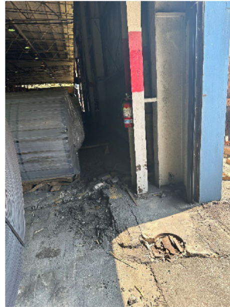
Photo 2.2.3.1.4 Slab failure with excessive settlement, cracking and spalling along West elevation at overhead door.
