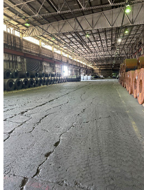
Photo 2.2.1.1.2 East bay steel truss framing to wide flange steel columns. Minor corrosion at base of exterior columns, remainder in good condition. Clean and paint all exposed steel
