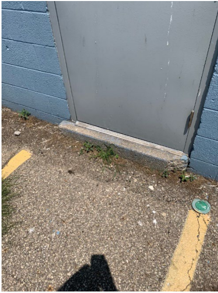
Photo 2.1.1.3.1 Hollow metal door at the Office face sheet has oil canning and the paint has faded. There is also a small step at the door that presents a tripping hazard.
