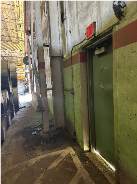
Photo 2.2.3.1.3 Slab failure with excessive settlement along West Elevation
