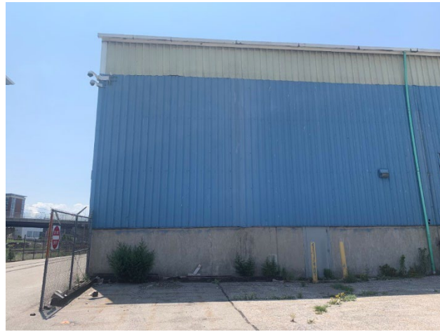
Photo 2.1.1.4.2 Translucent fiberglass clerestory panel at the top of the east wall of the warehouse. The panels are in fair condition. A portion of the panel on the left hand side is starting to pull away from the metal panel below.
