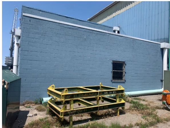
Photo 2.1.1.1.14 Mortar joints in the wall are worn and will need to be tuckpointed.
