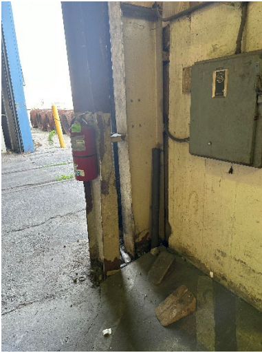
Photo 2.2.1.1.9 Minor rusting at base of columns along exterior elevation – Clean per SSPC-3 minimum and paint
