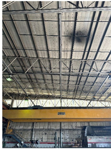
Photo 2.2.1.1.6 Existing Strut spanning from bottom chord between trusses damaged at train bay. Replace strut.
