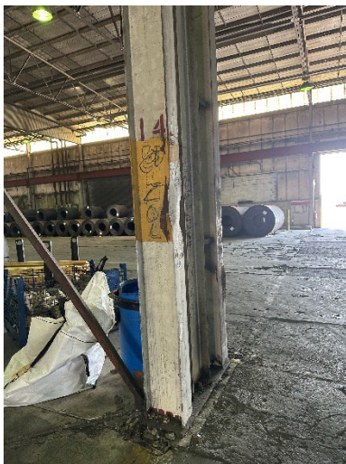
Photo 2.2.2.1.3 Existing crane column in center bay damaged by impact load
