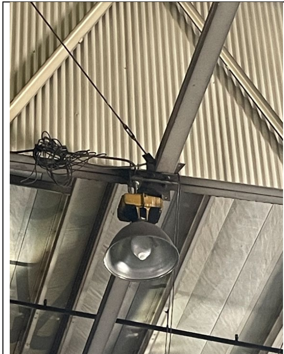
Photo 2.4.3.3 Close up of high bay lighting showing mounting to overhead electrical wireway
