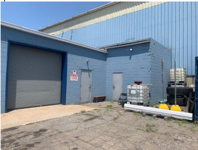
Photo 2.1.1.1.15 Areas of the CMU wall is heavily weathered and will need to be replaced. Lintels over the doors have started to fail and will need to be replaced and step cracking emanating from the corner will need to be repaired.
