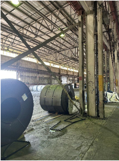
Photo 2.2.2.1.5 Existing angle x-bracing between crane columns bent/damaged.
