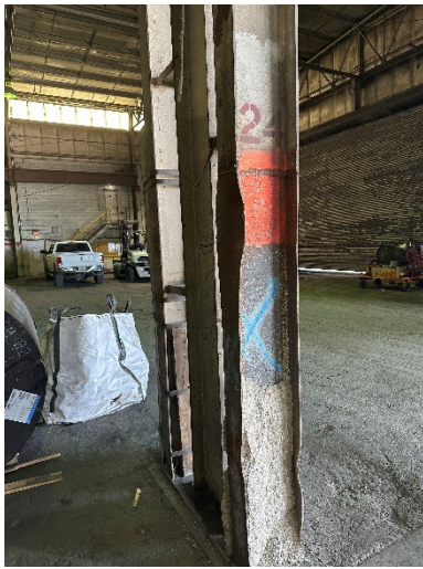
Photo 2.2.2.1.1 Existing crane column in center bay damaged by impact load.
