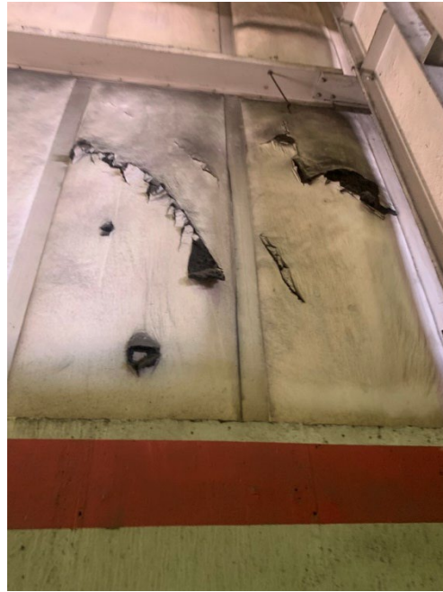
Photo 2.1.2.1.2 Scrim face on the batt insulation is damaged. Scrim face acts as the vapor barrier to stop water from entering the insulation and condensing causing damage.
