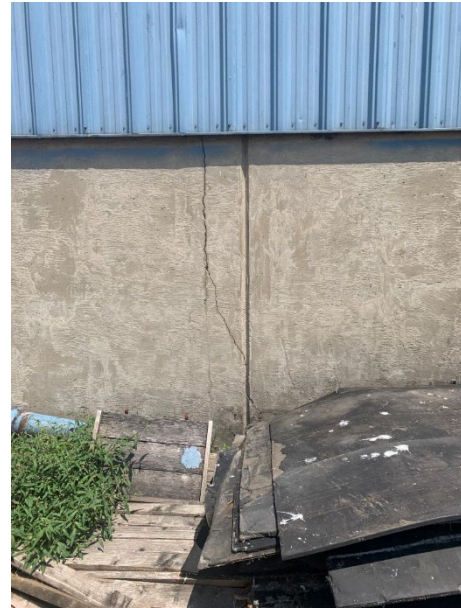
Photo 2.1.1.1.1 Vertical crack in the abuse wall.. Cracks should be routed out and repaired.
