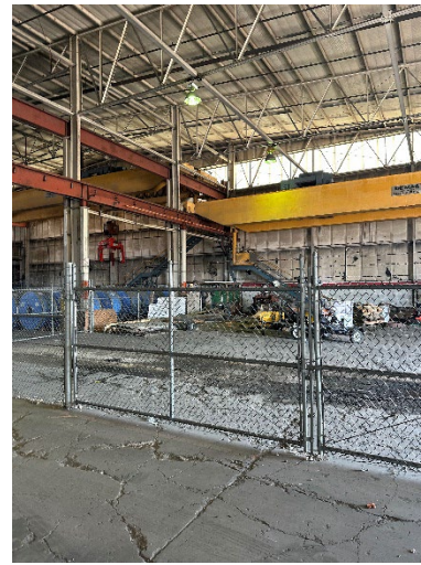
Photo 2.2.2.1.8 Existing crane in West bay not operational. Crane rail removed, crane girders and columns remain
