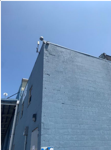
Photo 2.1.1.1.11 Heavily weathered CMU and mortar joints at the corner will need to be replaced. There are other areas in the CMU wall where the mortar joints will need to be tuckpointed.
