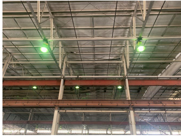
Photo 2.1.2.1.6 Scrim face on the batt insulation is damaged and falling away from the roof. Scrim face acts as the vapor barrier to stop water from entering the insulation and condensing causing damage.
