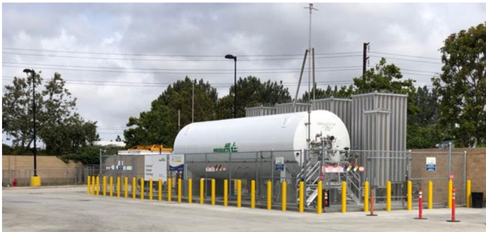
Figure E-3. Example of a liquid hydrogen refueling station
