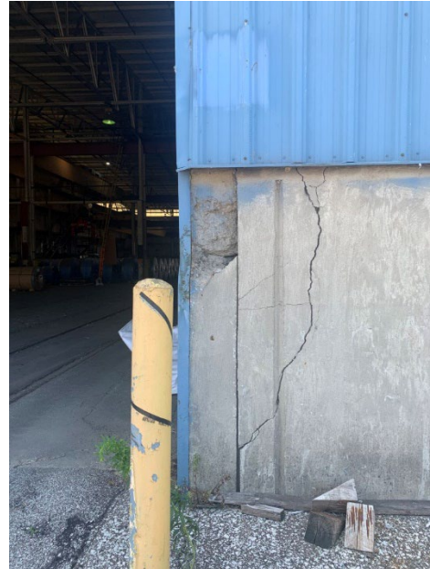
Photo 2.1.1.1.4 Vertical crack and large spalled area. Possible caused by a combination of differential settlement and impact damage.
