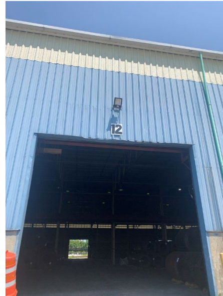
Photo 2.1.1.1.10 Damaged trim and metal wall panel at the head of the overhead door.
