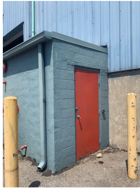
Photo 2.1.1.18 The central and southern sprinkler rooms are in fair condition and will require some minor masonry repair and tuckpointing of the mortar joints..
