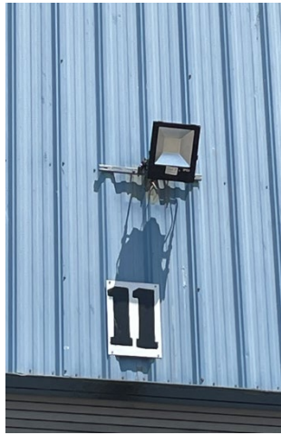
Photo 2.4.3.1 Close up of west side of Warehouse A showing LED wall pack used for area illumination
