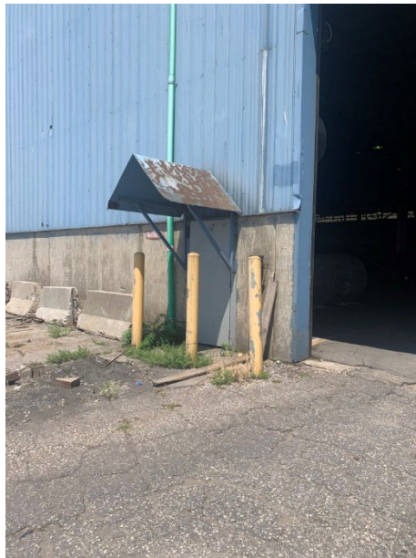
Photo 2.1.1.2.5 Canopy over existing door, is not original to the building construction and in poor condition. The paint on the canopy has failed and is beginning to corrode.
