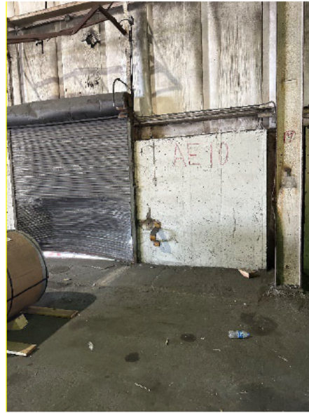
Photo 2.2.3.1.2 Slab failure with excessive settlement along East elevation
