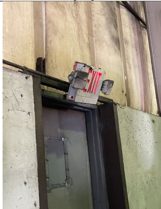
Photo 2.4.3.2 Exit sign on east side of Warehouse A. Damage shown here is typical of most exit doors.
