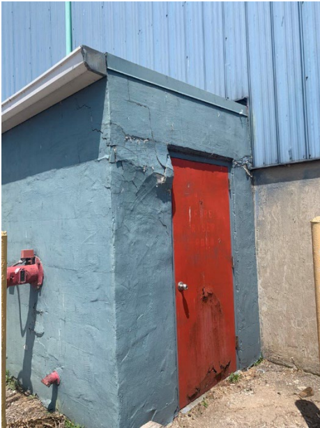
Photo 2.1.1.17 Northern Sprinkler roof CMU is in poor condition and has failed. The entire sprinkler room will need to be reconstructed.
