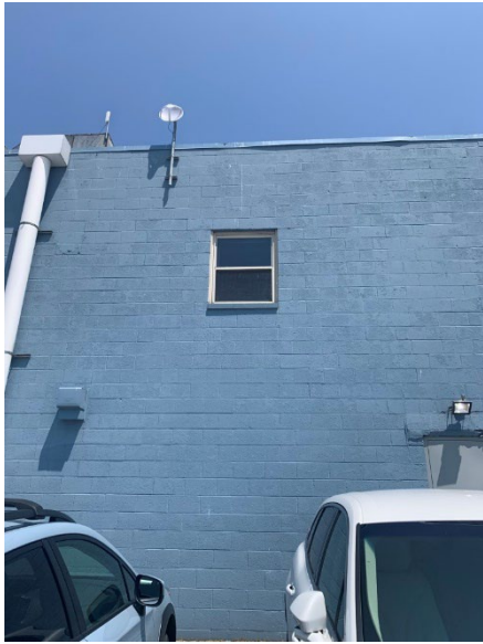
Photo 2.1.1.4.3 Office windows have been replaced and are in good condition. Sealant joints around the perimeter have reached their useful life and will need replaced.
