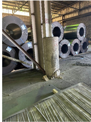
Photo 2.2.1.1.10 Existing concrete encasement at various crane/building columns damaged. Remove encasement and provide new concrete encasement at all column/crane columns to remain.
