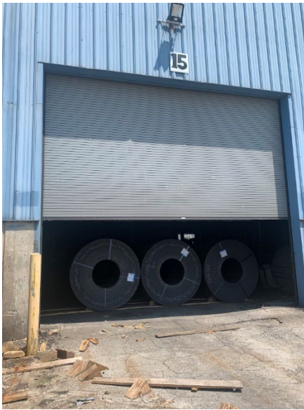
Photo 2.1.1.3.5 Some of the existing overhead doors are in fair to good condition. There is some minor damage on the slates but the door is operating.
