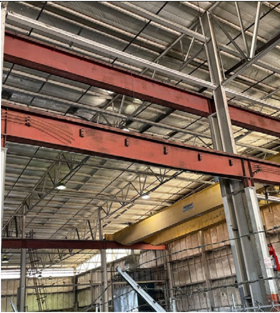
Photo 2.4.2.11 View of side of support beam on west side of Warehouse A, showing where crane busway has been removed
