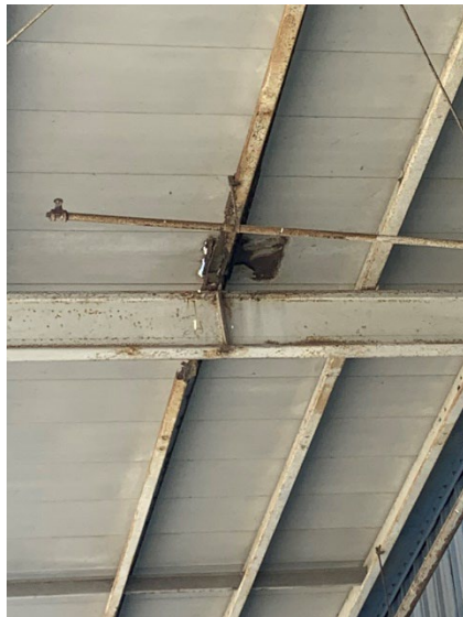
Photo 2.1.1.2.4 Underside of canopy over the dock area on the north side of the building. The structural standing seam deck is in poor condition with holes caused by corrosion.
