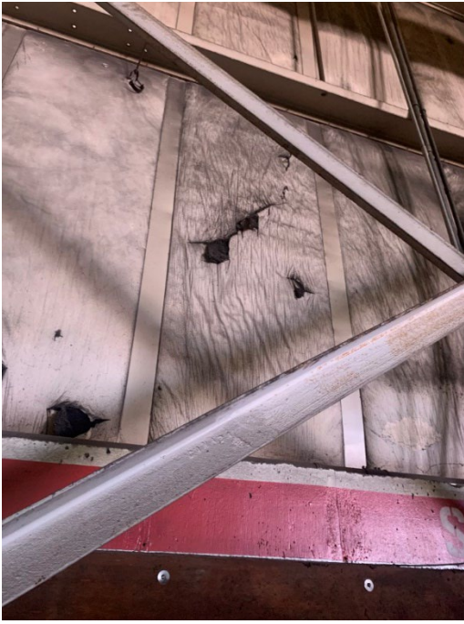
Photo 2.1.2.1.1 Scrim face on the batt insulation is damaged. Scrim face acts as the vapor barrier to stop water from entering the insulation and condensing causing damage.
