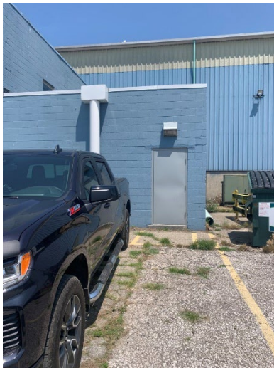
Photo 2.1.1.1.13 Lintel over the door is failing and will need to be replaced. Mortar joints around the lintel will need to be tuckpointed.
