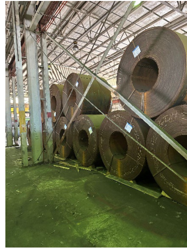
Photo 2.2.2.1.6 Existing angle x-bracing between crane columns bent/damaged. Existing rod x-bracing between building columns loose.
