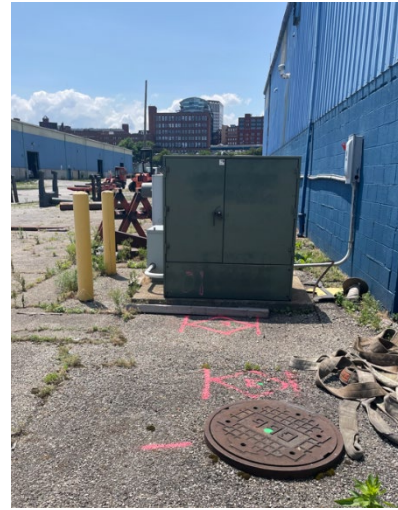
Photo 2.4.1.2 One of several CPP vault between W 3 rd St and Warehouse A, used for 2.4kV primary feed to site
