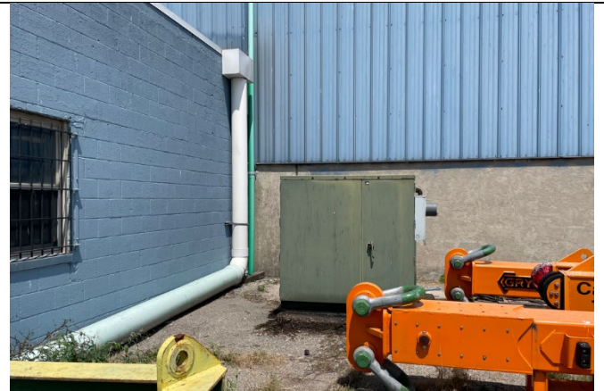
Photo 2.4.1.4 Location of utility transformer currently providing 480V power to Warehouse A
