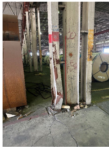
Photo 2.2.2.1.4 Existing crane column in East bay damaged by impact load
