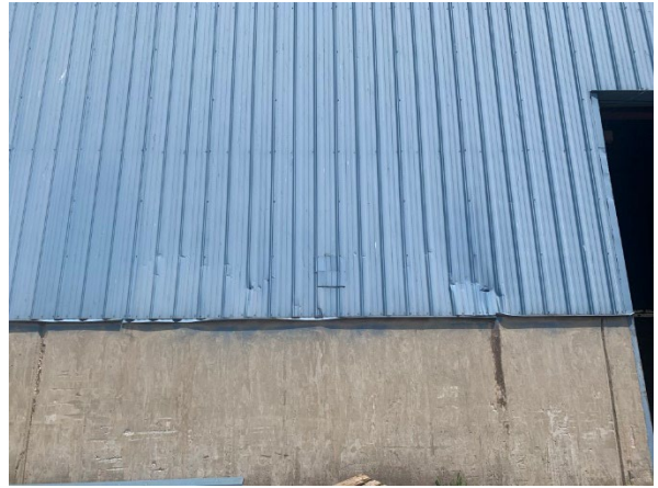
Photo 2.1.1.1.6 Damaged metal wall panels with dents and holes.
