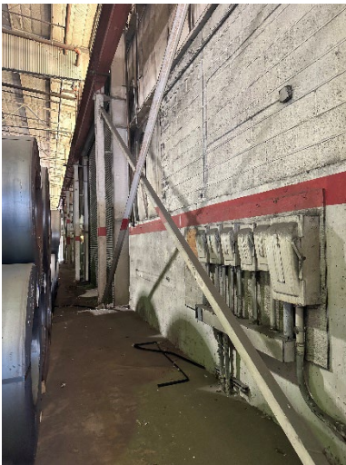
Photo 2.2.2.1.7 Minor rusting at base of columns along exterior elevation – Clean per SSPC-3 minimum and paint
