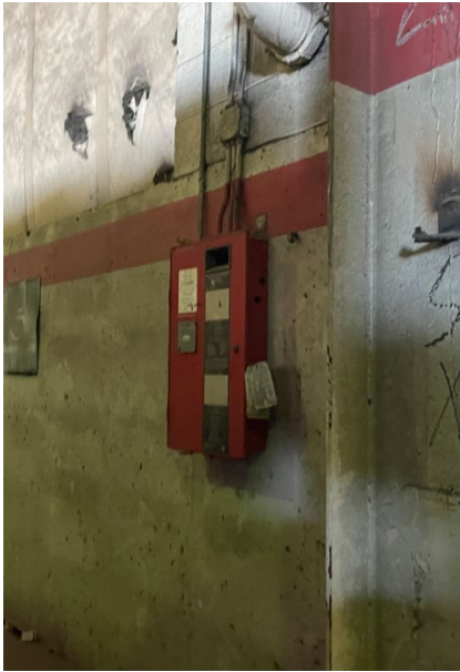
Photo 2.4.4.1 Non-functioning fire alarm control panel located at west side of Warehouse A
