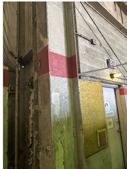
Photo 2.2.1.1.4 X-Bracing located on West elevation. 3/4" diameter rod bracing loose. Retention all rod x-bracing.
