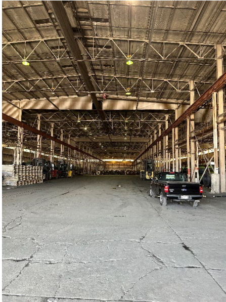
Photo 2.2.1.1.1 Center bay steel truss framing to wide flange steel columns at 24'-0" on center. Steel trusses and interior columns in good condition. Clean and paint all exposed steel.
