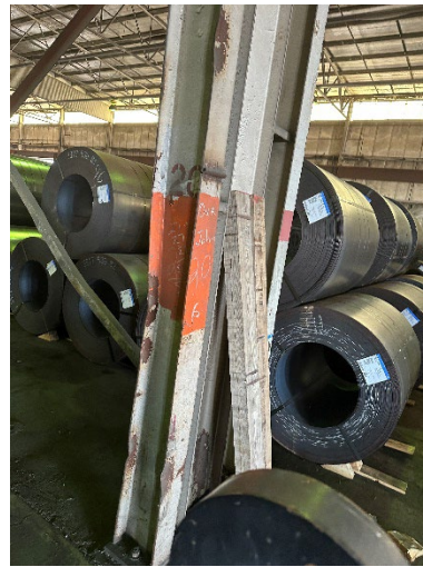
Photo 2.2.2.1.2 Existing crane column in center bay damaged by impact load
