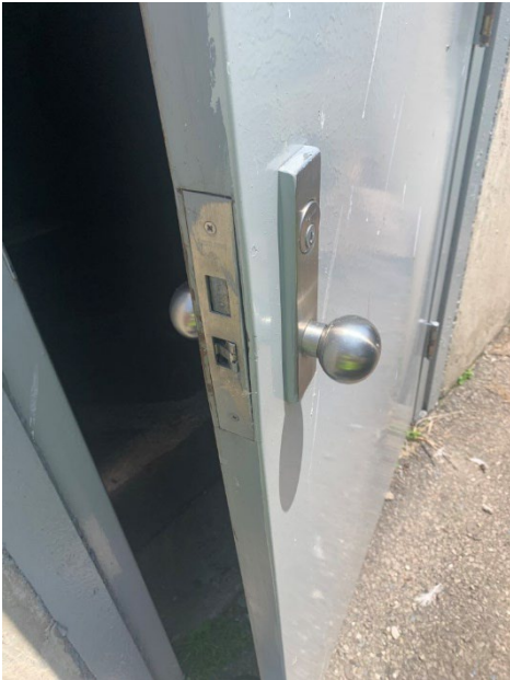
Photo 2.1.1.3.3 Door hardware is not functioning properly with closers and locksets not working. Additionally doors are provided with knob handles and not levers as required by ADA.
