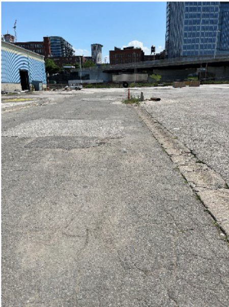
Photo 3.1.1 Pavement along west side of the warehouse and roadway with concrete curb (photo looking south).
