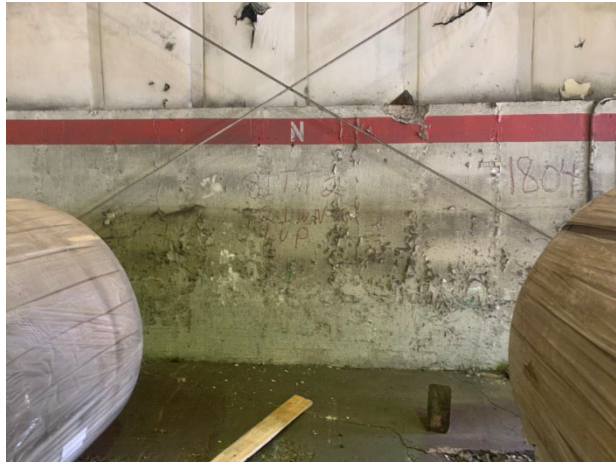
Photo 2.1.2.1.4 Paint and coating on the concrete abuse wall is failing and peeling.
