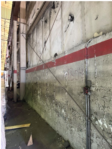
Photo 2.2.1.1.5 X-Bracing located on West elevation. 3/4" diameter rod bracing loose. Retention all rod x-bracing.
