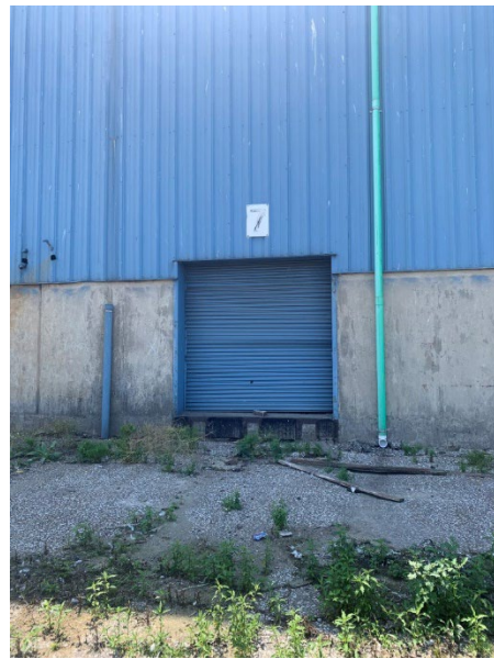
Photo 2.1.1.3.6 Overhead door is in poor condition and does not operate correctly. Door slats are damaged.
