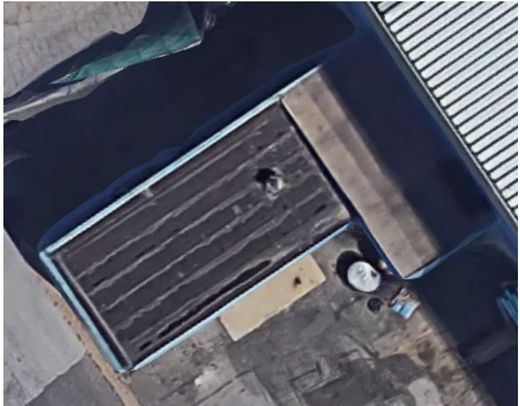
Photo 2.1.1.2.3 Aerial image of the Substation roof. Existing roof appears to be a built-up modified bit roof. Areas of asphalt flowing from under the plies is observed.
