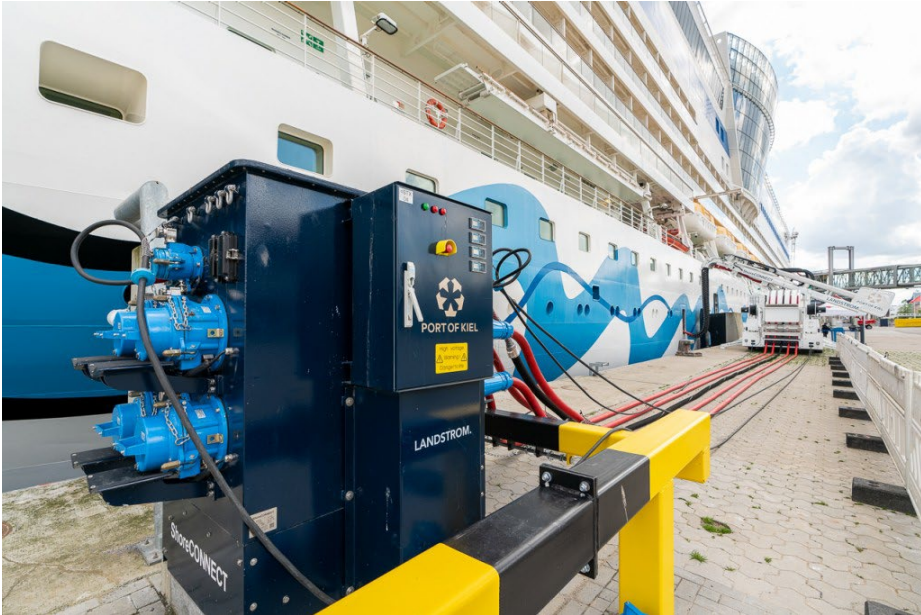
Figure I-7. Example Above Grade Electrical Connection
