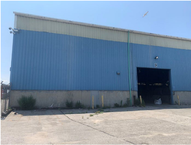
Photo 2.1.1.1.5 Existing metal siding is faded and has differently coloration and staining.
