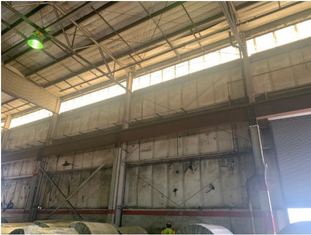
Photo 2.1.2.1.3 Scrim face on the batt insulation is damaged. Scrim face acts as the vapor barrier to stop water from entering the insulation and condensing causing damage.
