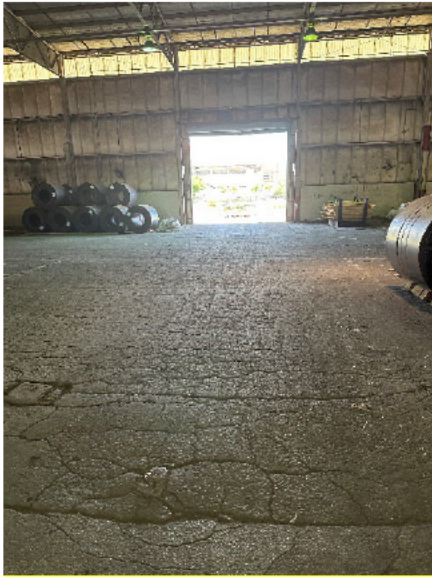
Photo 2.2.3.1.1 Typical slab concrete cracking throughout entire surface of building
