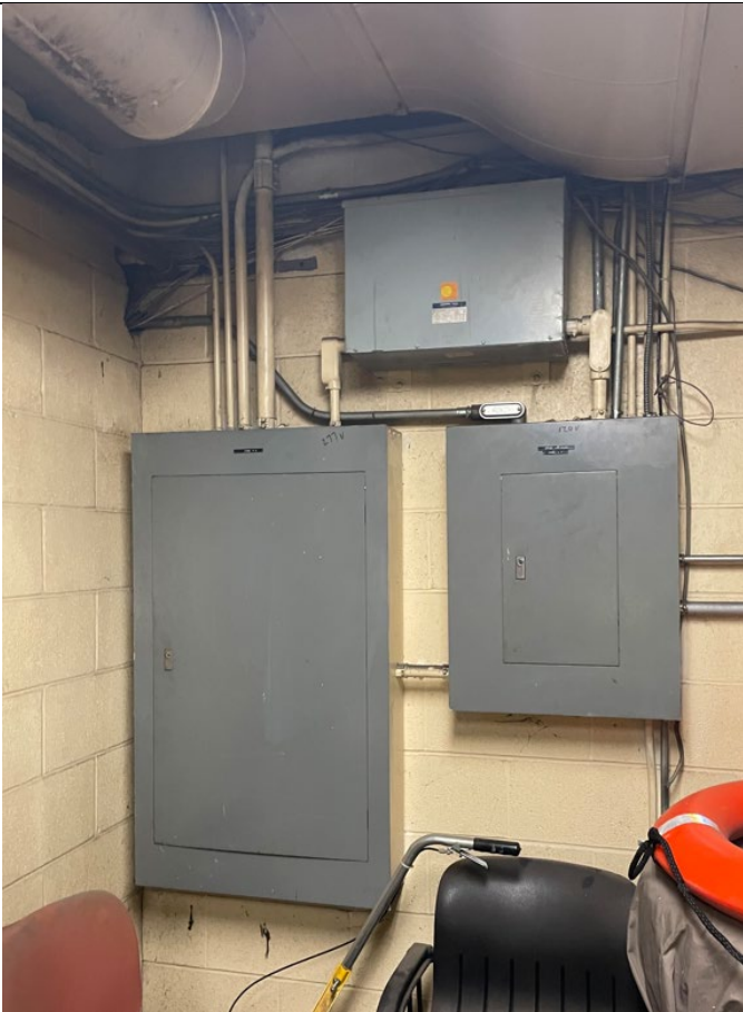
Photo 2.4.2.13 Panelboards serving two story office on east side of Warehouse A appear to date to 1970s era construction
