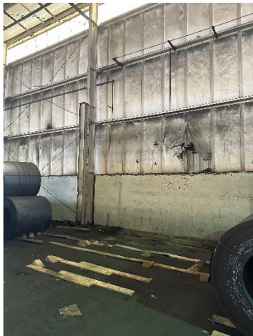
Photo 2.2.1.1.7 Typical girt framing along East elevation in fair/good condition. Clean and paint
